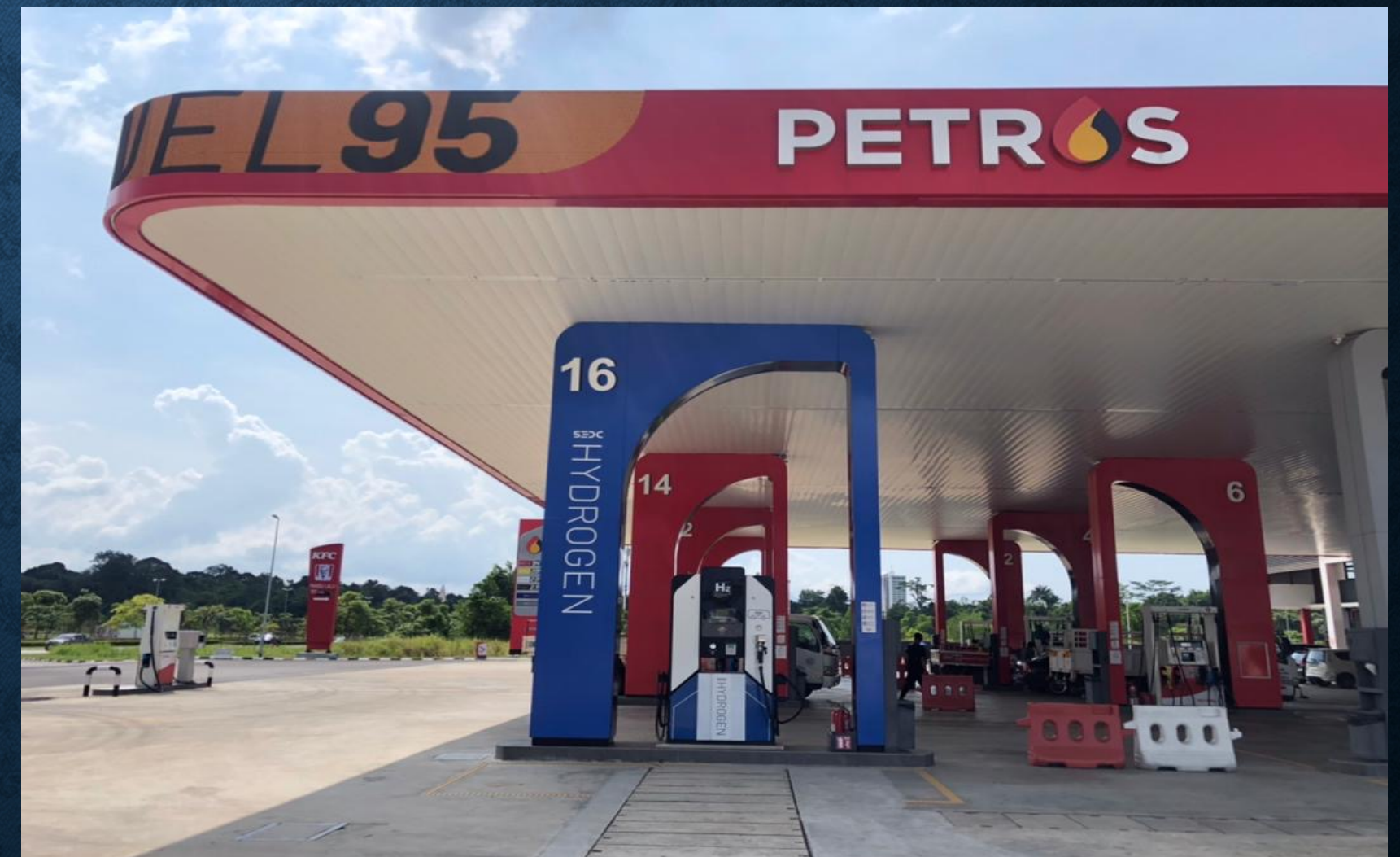
H2 Refuelling Station at Petros Darul Hana
