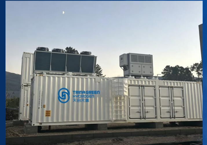
Hydrogen production and refueling integrated station Portugal, Europe
